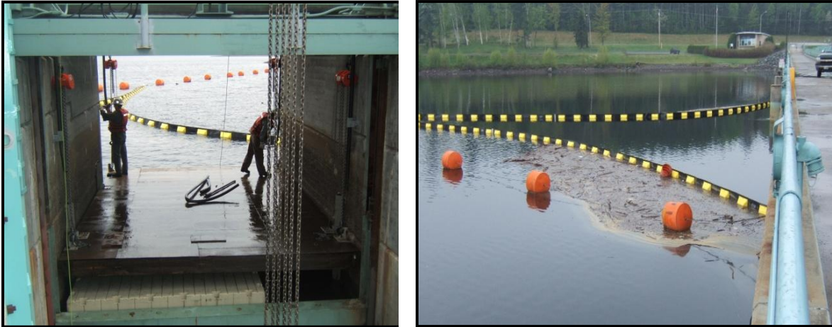
Figure 2-3. Moore fish trap attraction flow shelf raised for repairs (left), view is looking upstream through the skimmer gate entrance to Moore Reservoir; and the debris boom (right).
