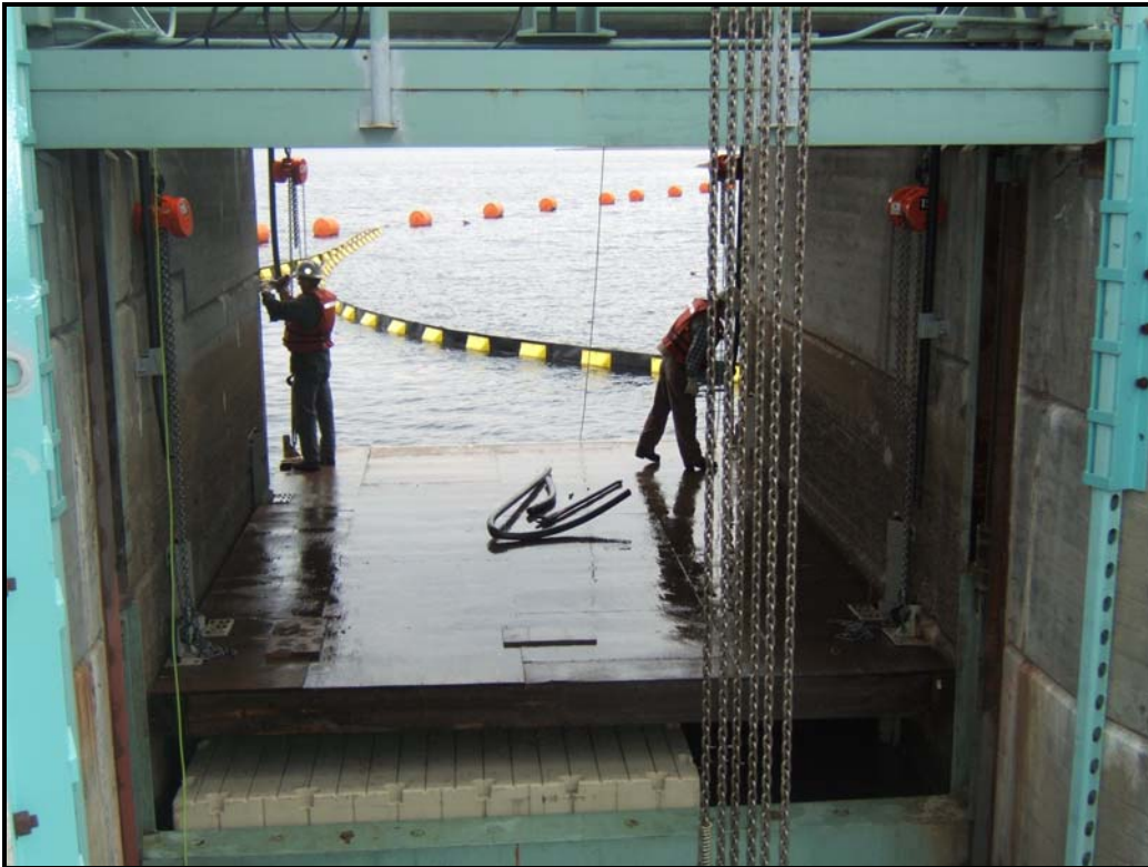
Figure 2-5. Moore Development, attraction flow shelf raised for repairs. View is looking upstream through the skimmer gate entrance to Moore Reservoir.
