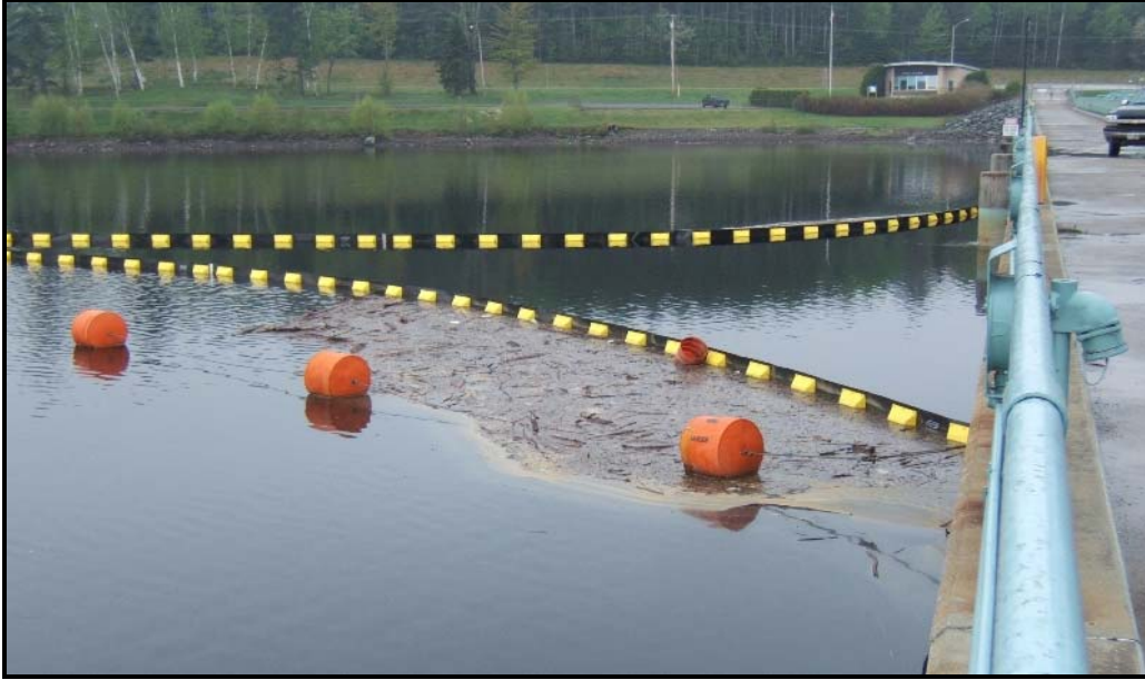
Figure 2-6. Moore Dam trash boom installed at the entrance to the skimmer gate.
