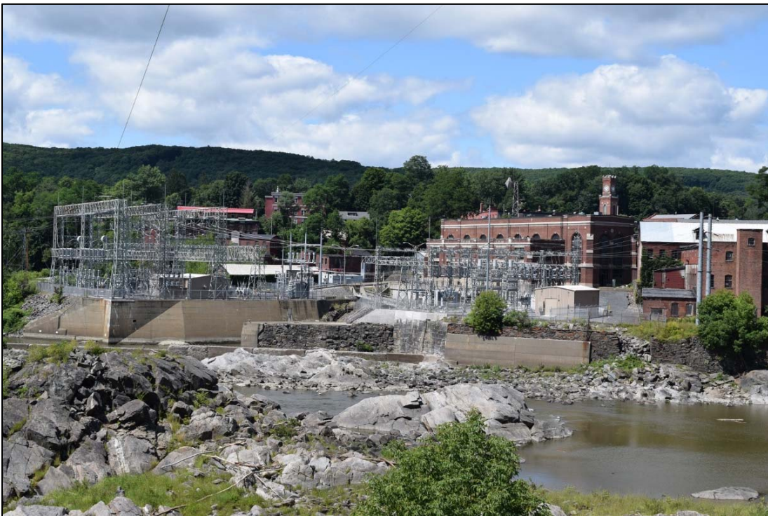
Photo 5-2. Bellows Falls Project, general view of Powerhouse, Tailrace, and Switchyards at south end of Bellows Falls Island, looking west from New Hampshire shoreline.
