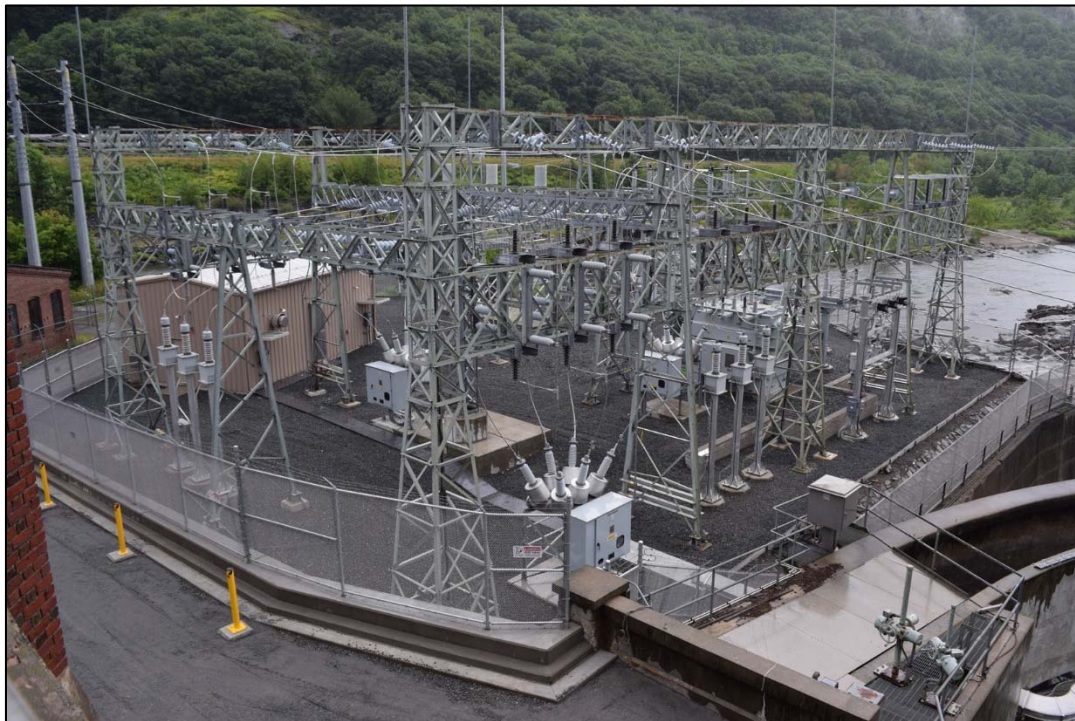
Photo 5-13. Bellows Falls Project, 6 & 69 kV Switchyard, looking southeast.
