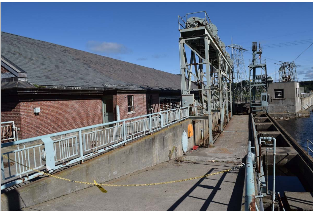
Photo 4-5. Wilder Project, Dam at Powerhouse substructure with east elevation of Powerhouse, looking north.
