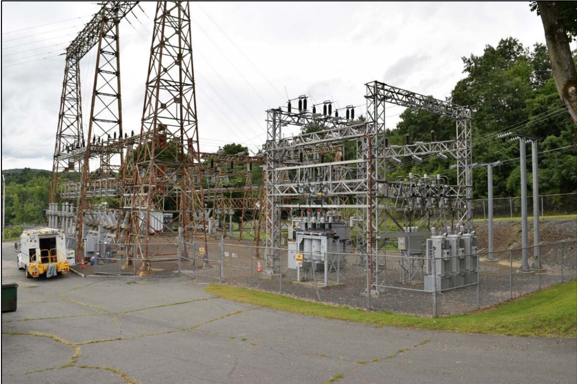
Photo 6-10. Vernon Project, Switchyard, looking southwest.
