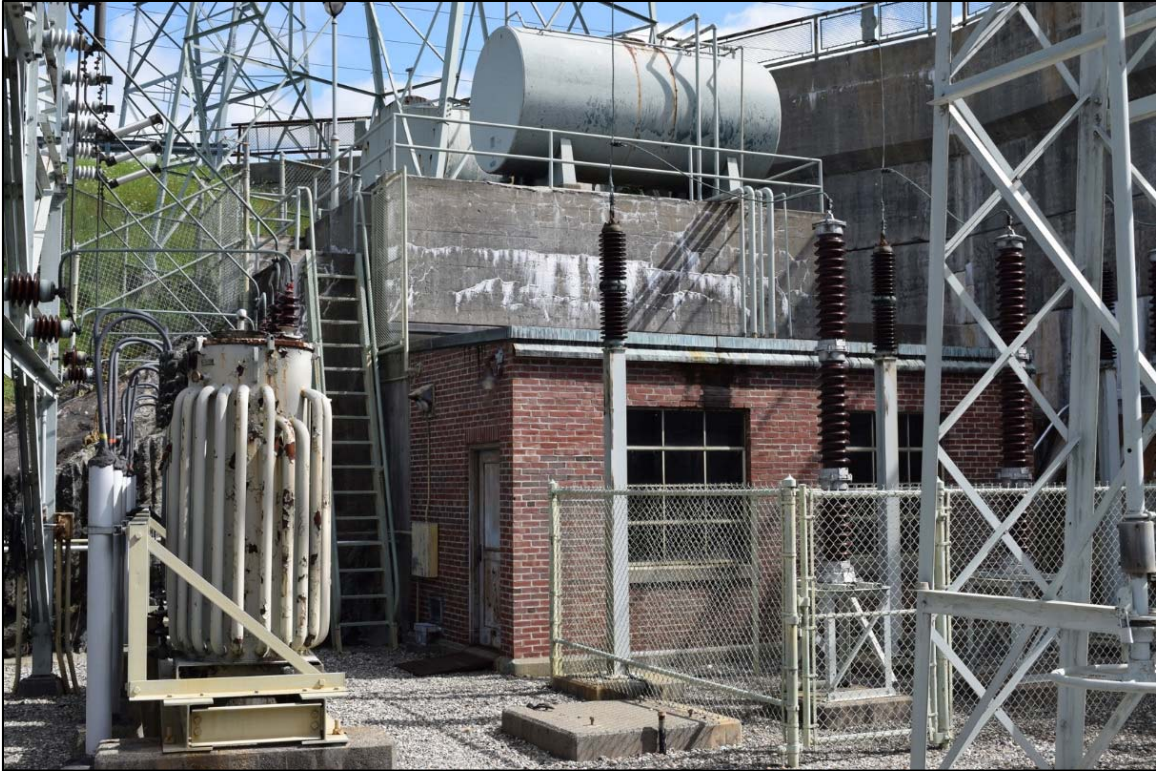
Photo 4-13. Wilder Project, Oil Pump House within 13.8-, 47-, & 115- kV Switchyard, looking north.
