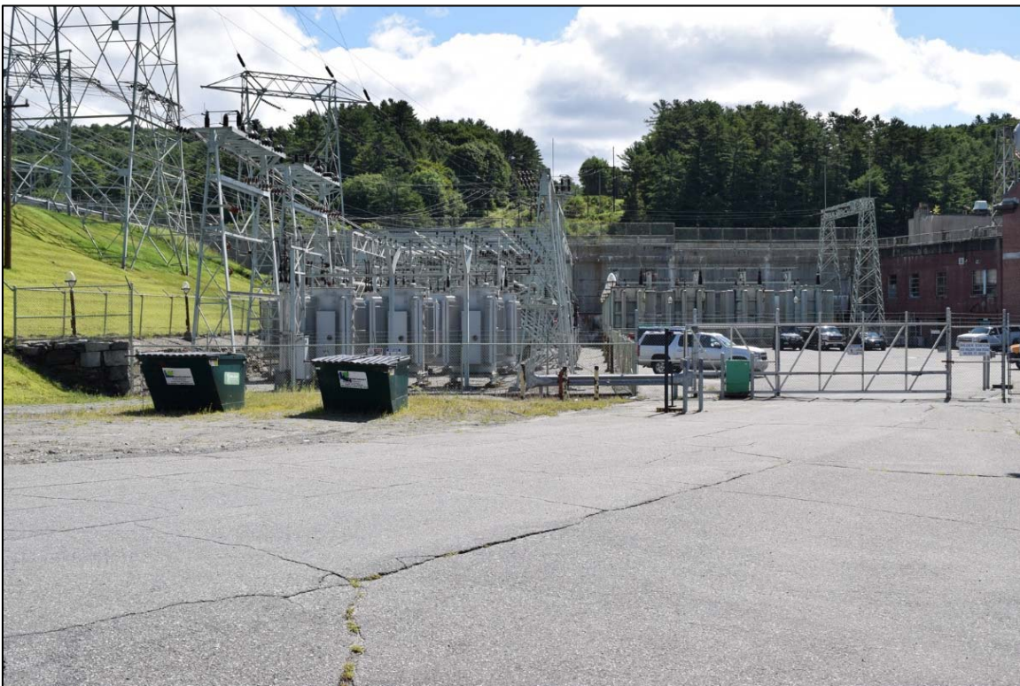
Photo 4-12. Wilder Project, TransCanada 13.8-, 47-, & 115-kV Switchyard, looking southeast.
