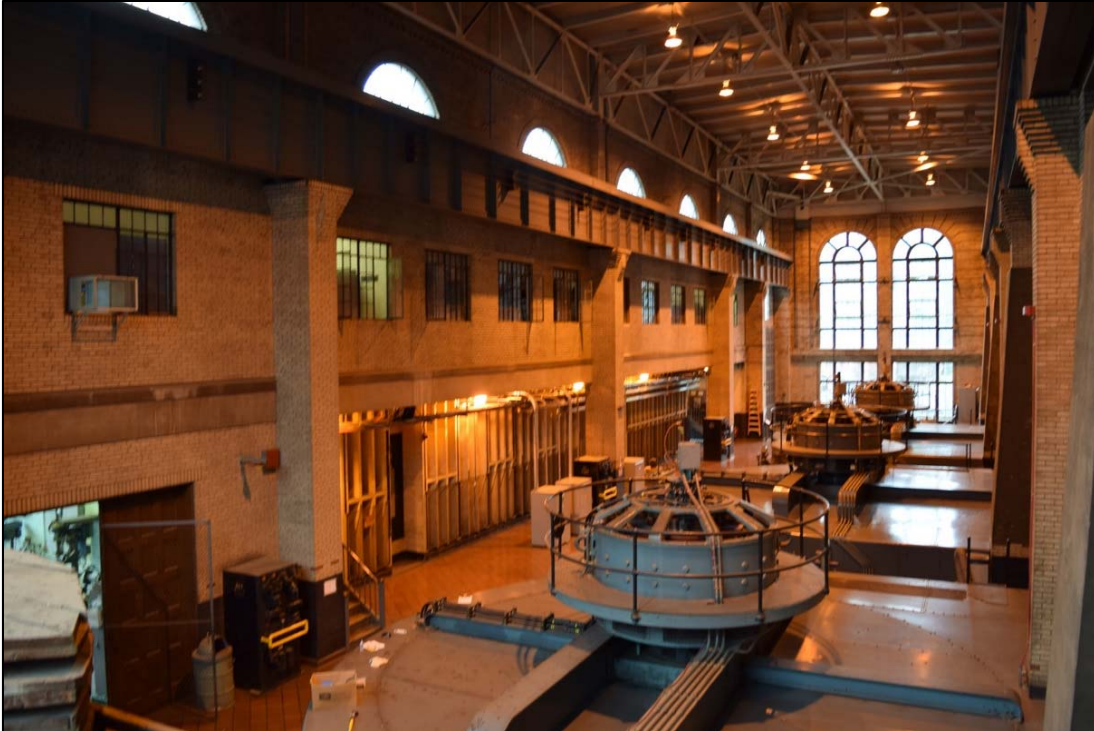
Photo 5-11. Bellows Falls Project, interior of Powerhouse generator hall.
