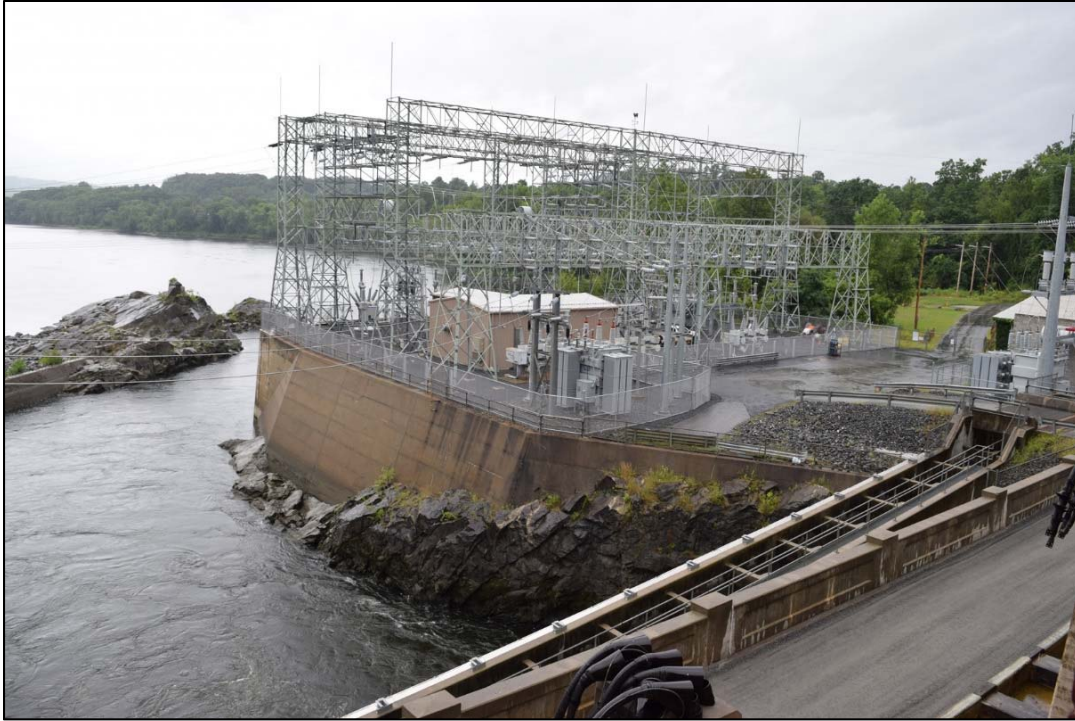
Photo 5-12. Bellows Falls Project, 115 kV Switchyard looking southwest.
