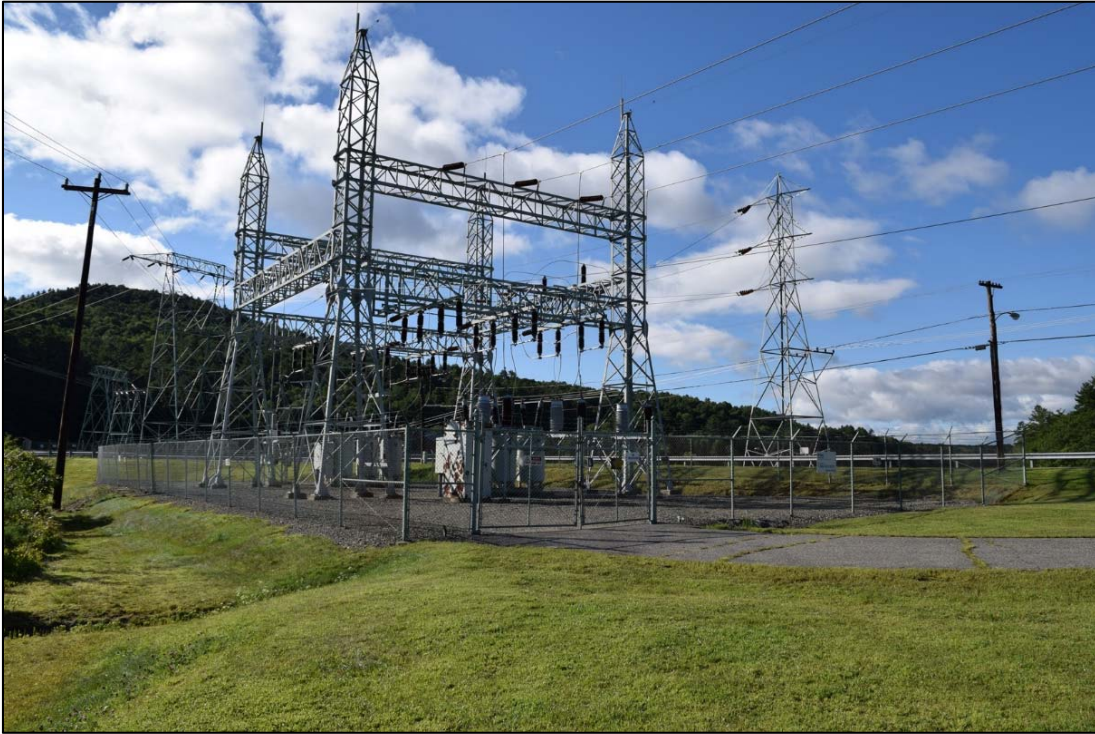
Photo 4-14. Wilder Project, National Grid 115-kV Switchyard, looking south.
