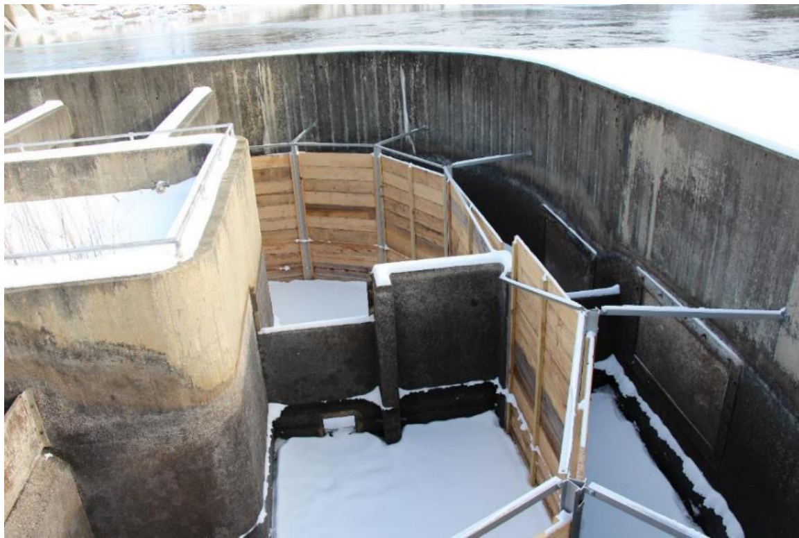
Figure 3.6-21 Partition wall installed at the Vernon fish ladder prior to the 2019 fish passage season.
