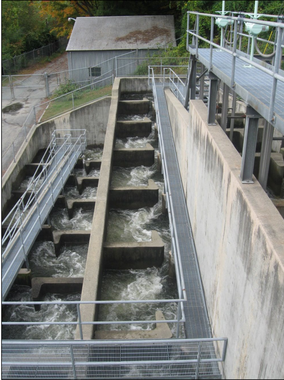
Figure A-9. Upstream fish passage facilities.
