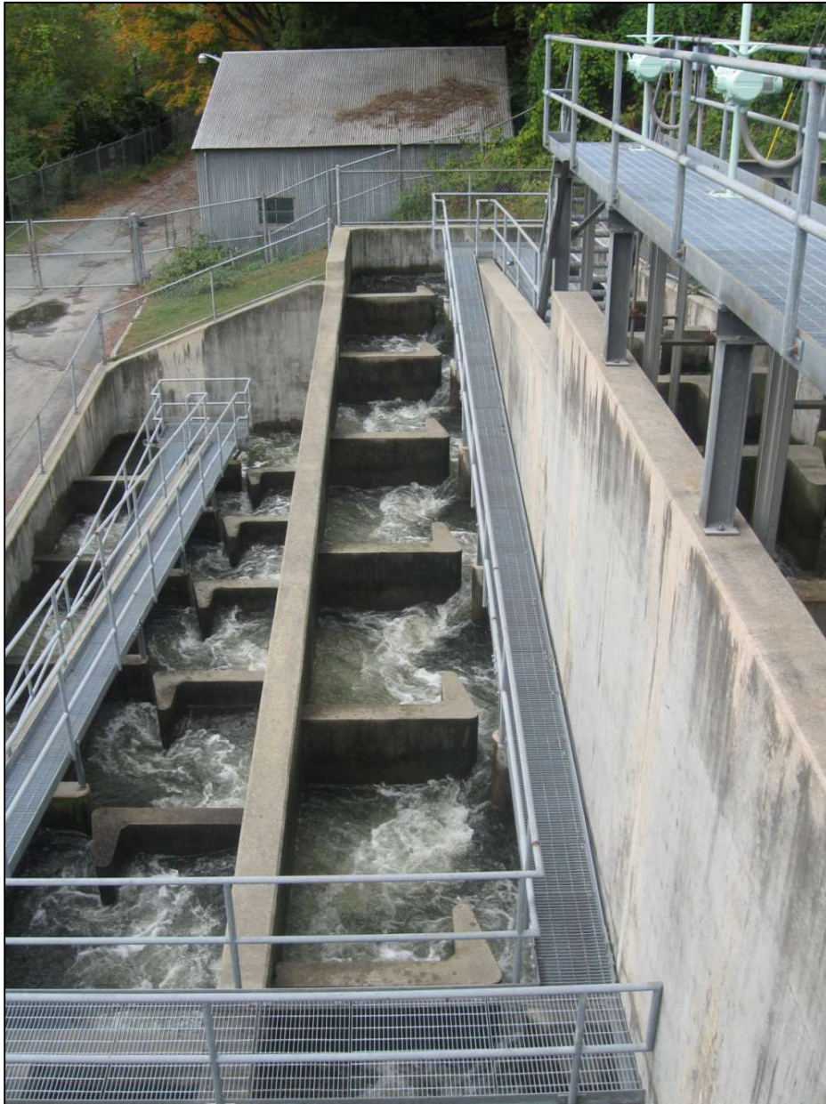
Figure A-9. Upstream fish passage facilities.
