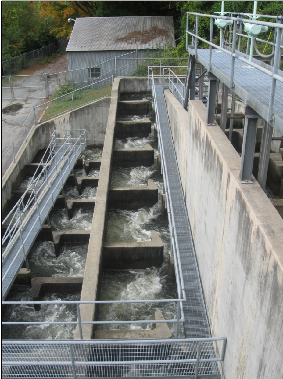
Figure A-9. Upstream fish passage facilities.
