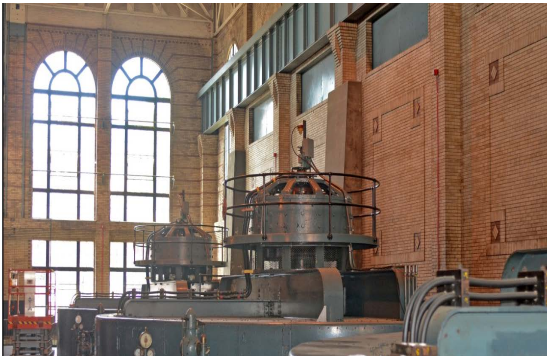
Figure A-6. Unit No. 1 (background) and Unit No. 2 (foreground).
