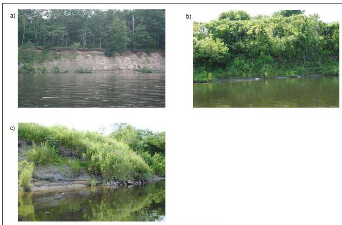
Photos of the unstable bank categories: a) eroding, b) vegetated eroding, c) failing armor.
