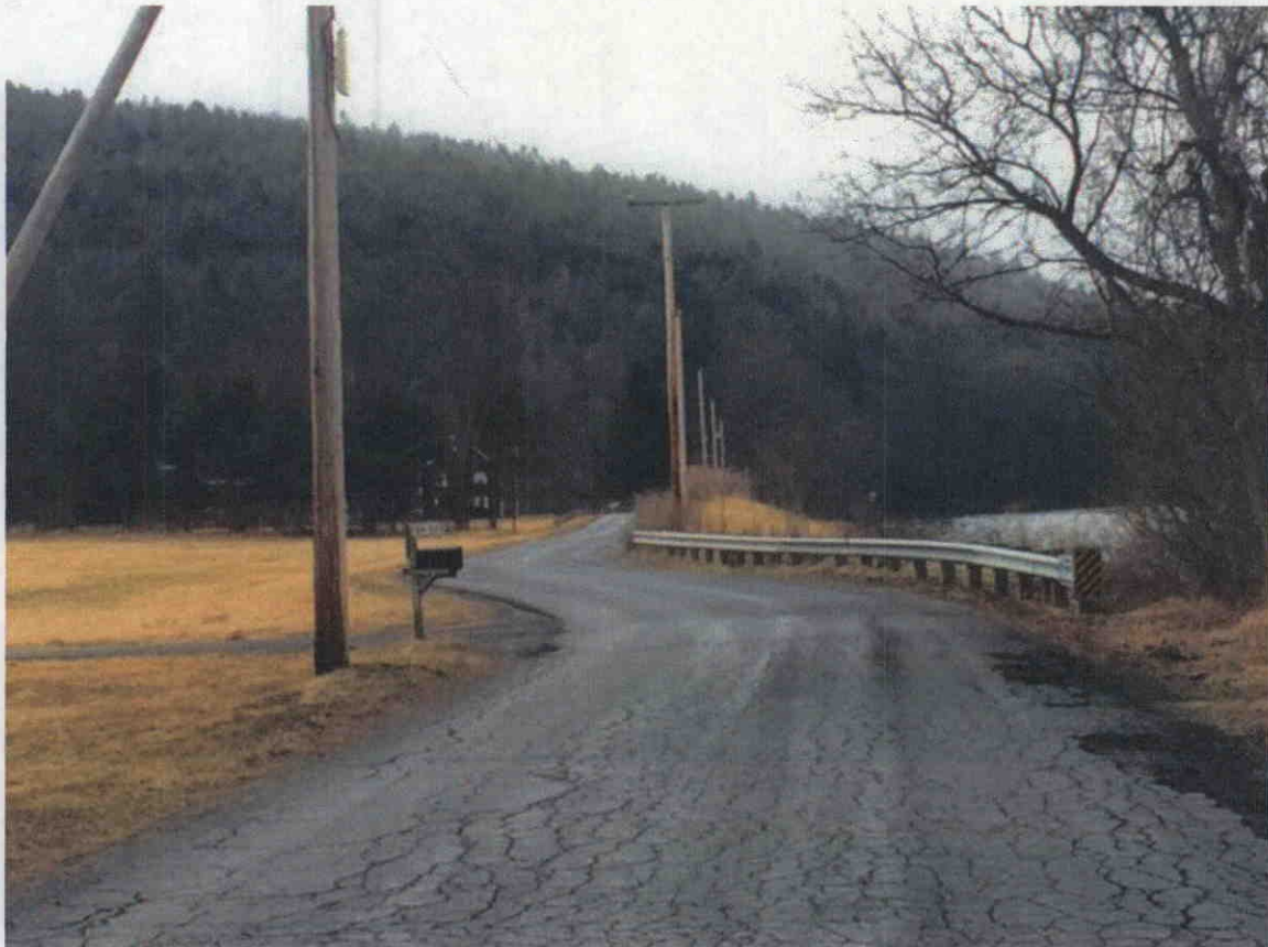
Fig4. This is the “dog leg” of the reconstructed road. It can be viewed from the river as well. Why was this change not noted on 2014 map of survey of erosion?
