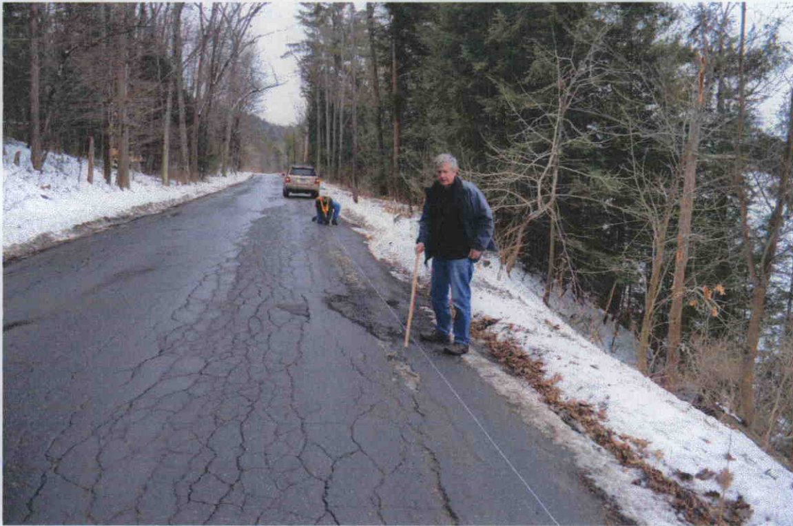
Figure 5. A photo taken in 2013 of River Road, Lyme, looking south about a quarter of a mile south of the East Thetford bridge. The string is on the road at each end of the slump which is 7 inches below the string in the center. Note the cracking of the blacktop on the west side of the road due to the slump and compare it with the linear cracking seen in the photo taken at the site of the collapse near the North Thetford road in Figure 2
