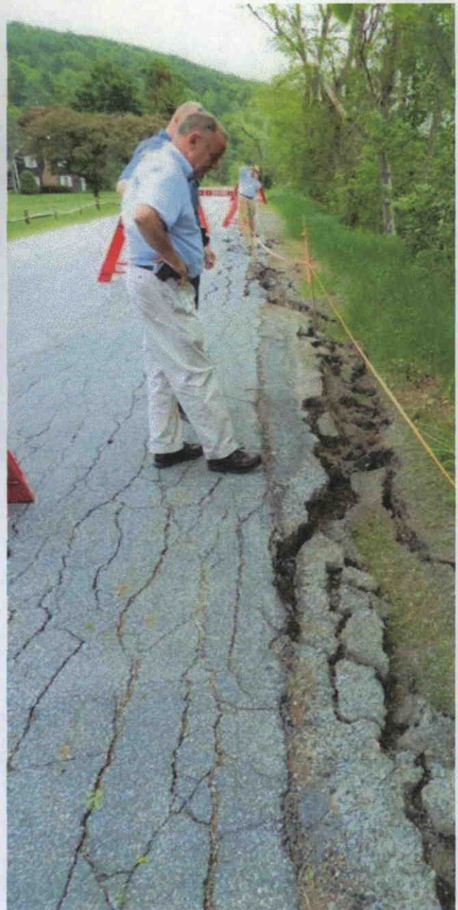
Figure 2 River Road north adjacent to bank collapse. Note pattern of cracks in blacktop and compare with those in photo X, below, in area of slumping River Road South.
