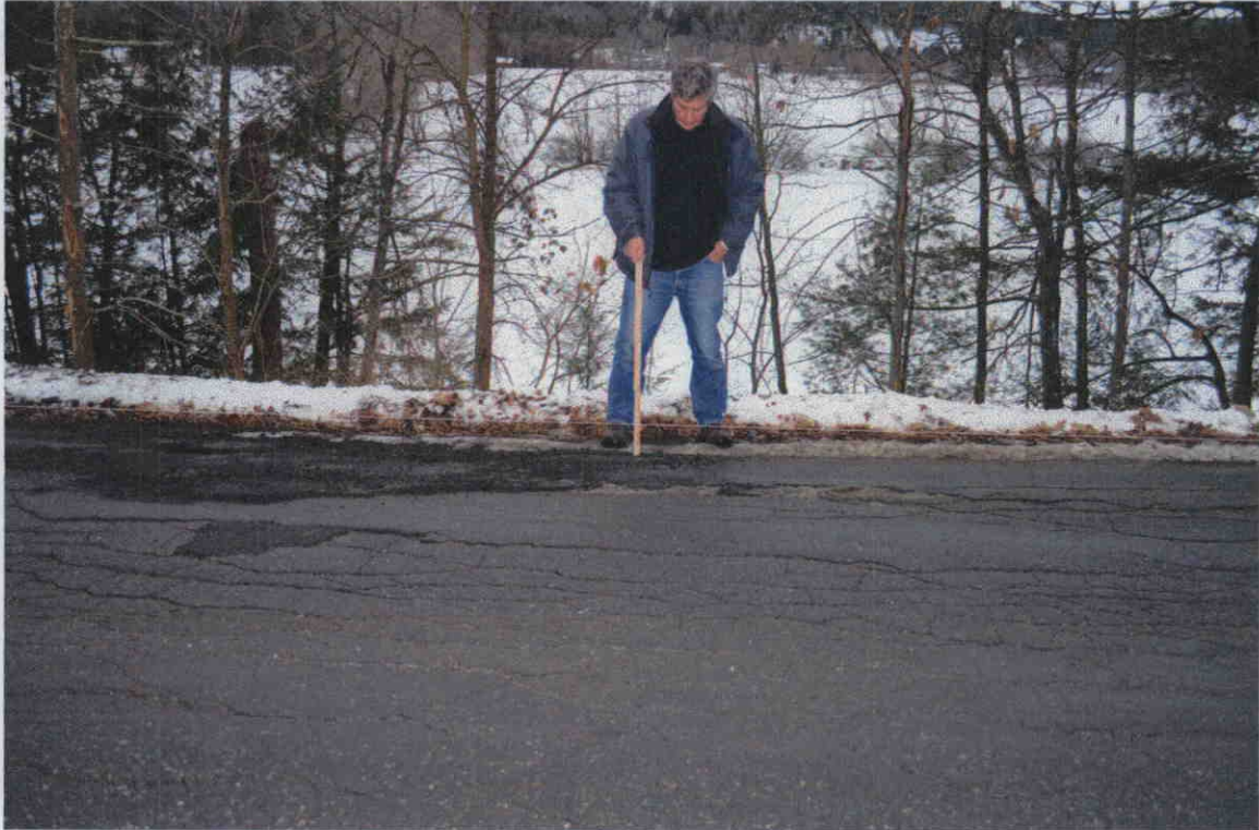
Figure 6. 2013 photo of River road south looking west. Wilder impoundment in background. Slump in road is 7 inches. In 2014 this slump had progressed alarmingly and catastrophic failure was felt likely by consulting engineers. The road has been closed for two years while plans for constructing a bypass are developed and financed. Cost estimates are in the $2 million range.
