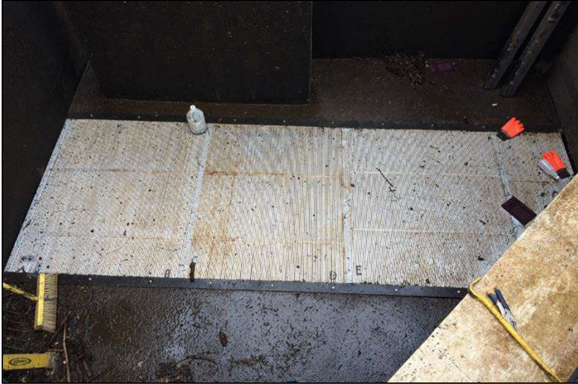
Figure 1.0-6. Aluminum dewatering screen on diffuser room floor.
