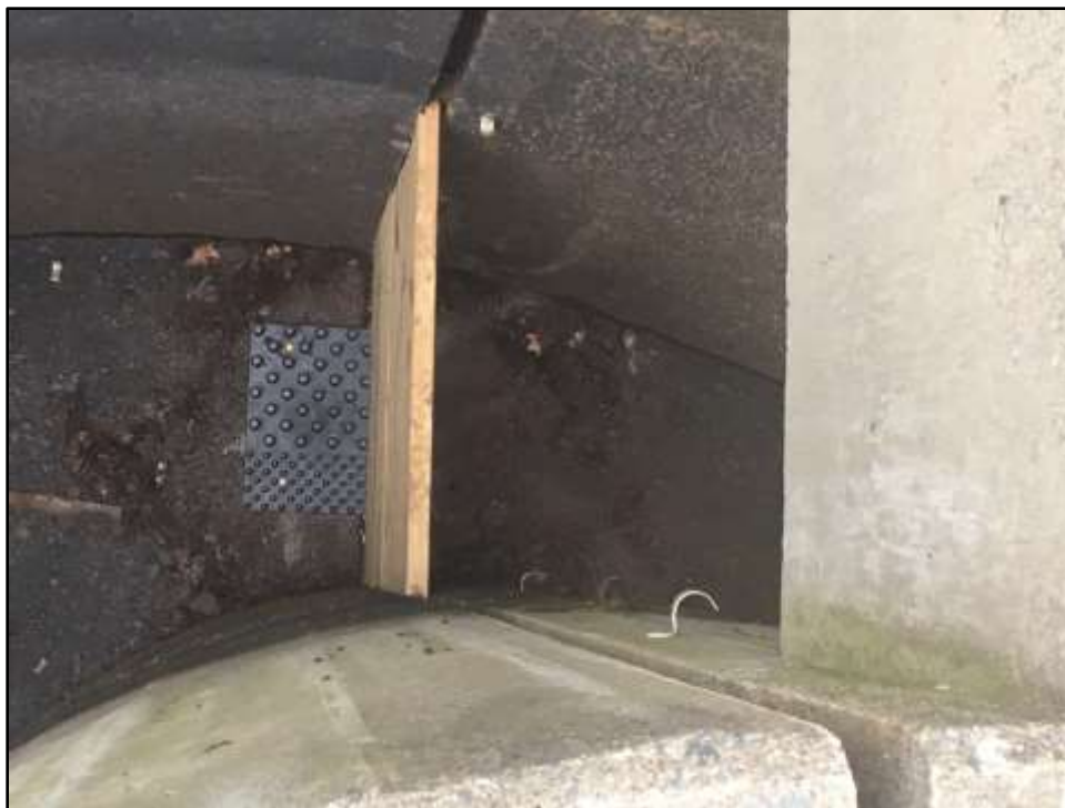
Figure 1.0-4. Exit Weir from above with eel tile and before upstream baffle installed.
