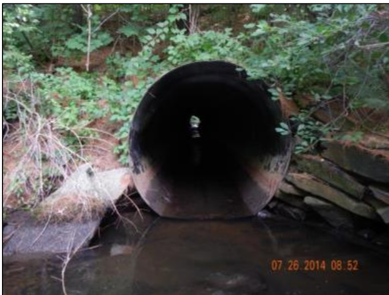
Culvert near upstream extent of project-affected area associated with Site CT-B-3.35 as determined by visual observations, 2014.
