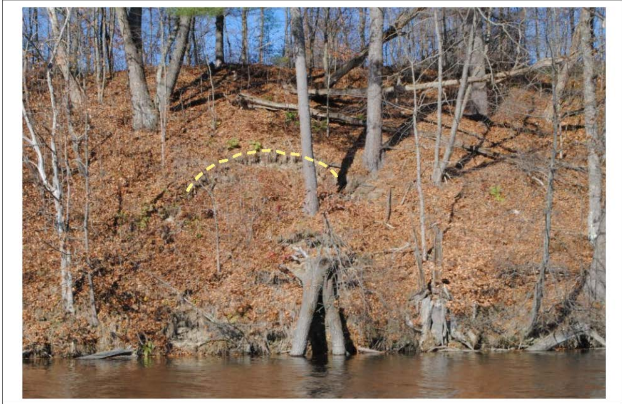
Figure 5.6.2-3. Active erosion can occur despite the presence of bank vegetation. Dashed yellow line outlines top of planar slip scarp.
