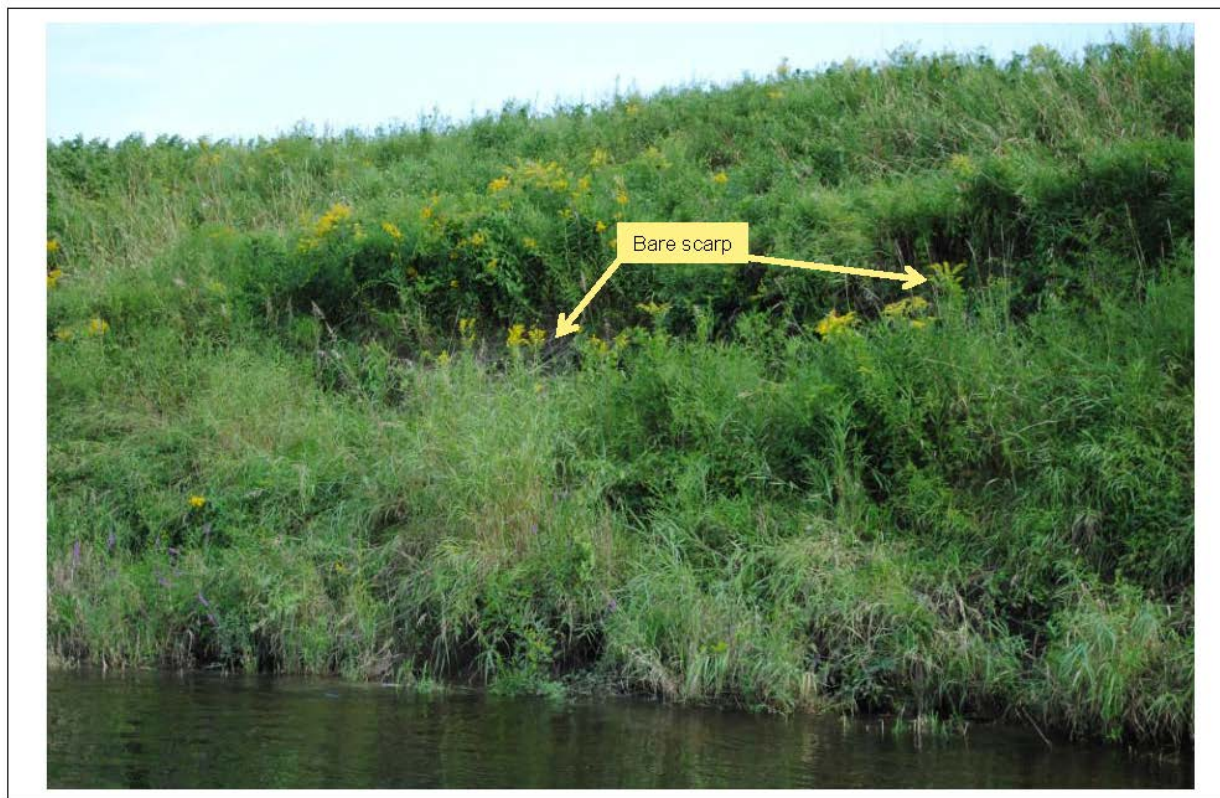
Figure 5.6.1-3. Sometimes barely visible scarps are the only evidence of active erosion on well vegetated banks.
