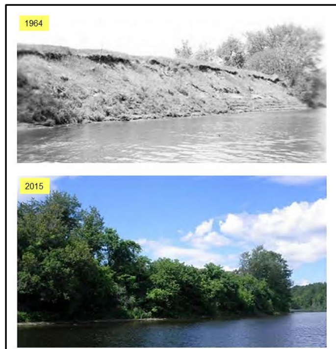
Figure 4. Eroding bank on Connecticut River in Bellows Falls Pool in 1964 was stable by 2015.
